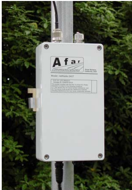
Figure 1.1. Pole Mounted Radio
